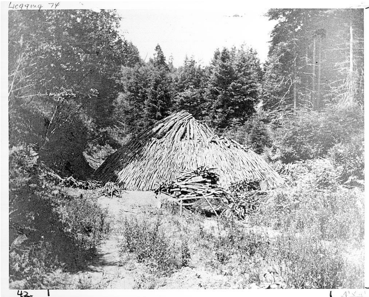
Charcoal mound under construction, Sonoma County, 1915 (Sonoma County History and Genealogy Library, Photo 29332)
